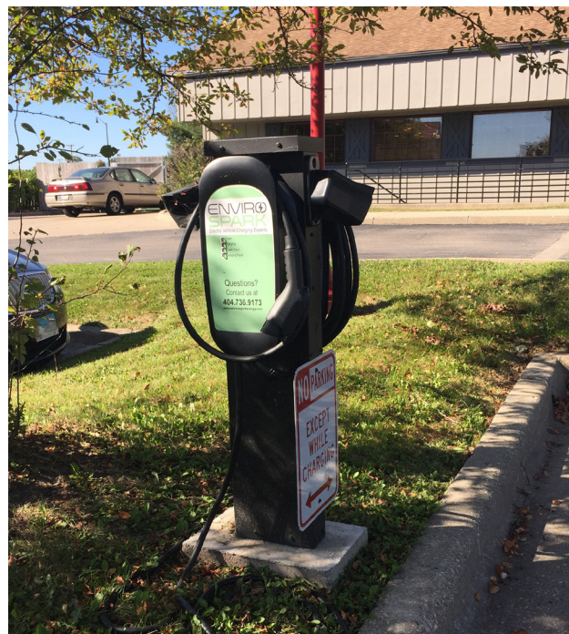
EV Charging Station at the Machine Shed. Rockford, IL.
