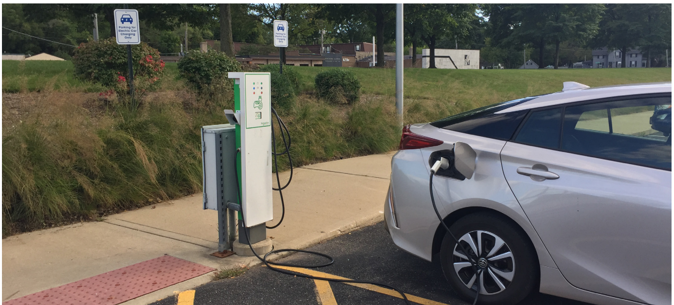
EV Charging Station at Nicholas Conservatory & Gardens. Rockford, IL.
