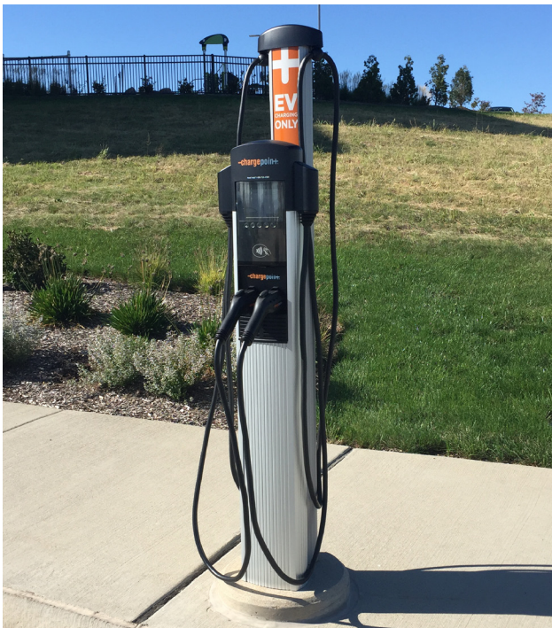
EV Charging Station, MercyHealth Medical Center, Rockford, IL.
