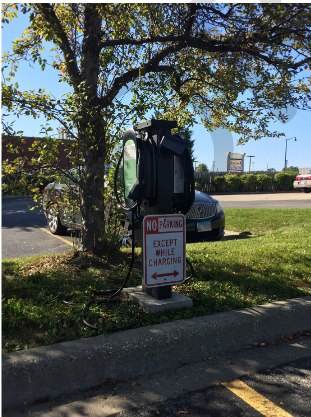
EV Charging Station at the Machine Shed. Rockford, IL.
