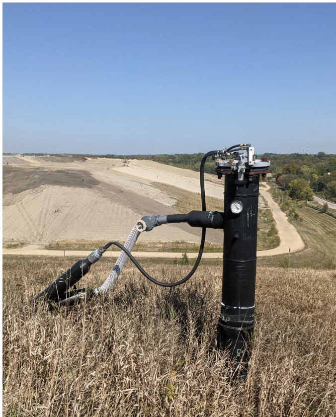
Landfill Gas Capture System Component in Winnebago County
